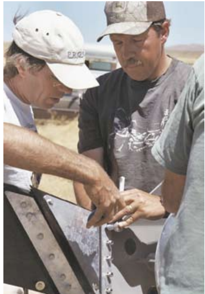
Installer Chris Worcester, and owner Paul Thomas attach blades to the Proven's downwind hub.
